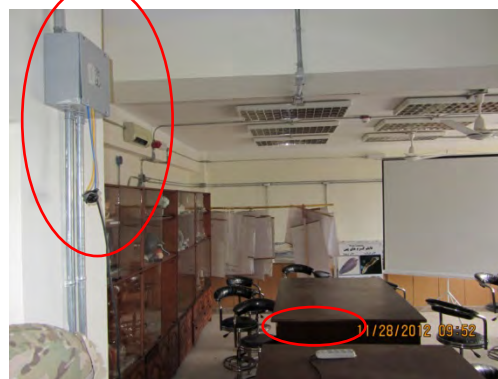
Photo 2 - Laboratory with Electrical Tap Visible from the Junction Box and Wire Leading to Power Strip
