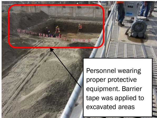
Figure 2 - Over-Excavation of Sewage Filter Beds
