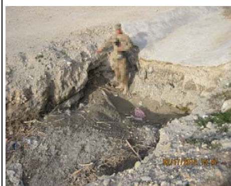
Storm Drain Erosion
