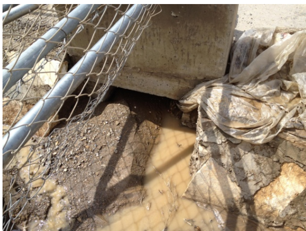
Figure 2 - Storm Water Ditch Clogged with Sediment
