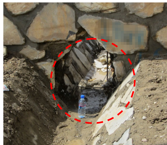
Figure 3 - Storm Water Ditch Missing Security Grate
