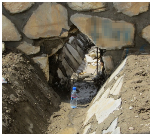
Missing Grate Could Allow Unauthorized Access
