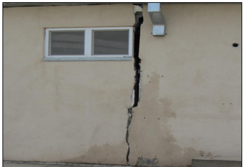
Exterior Structural Failure, Building 603 (latrine), Kunduz Army Garrison, March 2012
