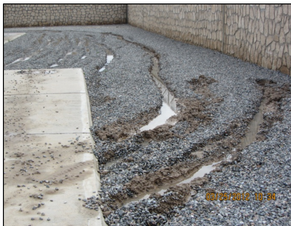
Figure 9 - Ruts from Off-Road Driving
