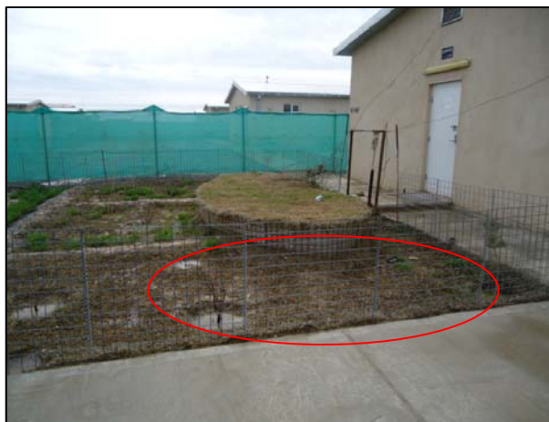
Figure 8 - Improper Grading and Landscaping
