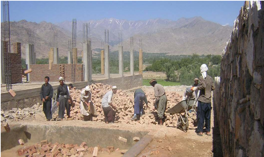
Site Photo 3: Laborers working to complete the Kohi Girls' School in August 2009. Projects such as this one provide legitimate local employment while allowing workers to develop new skills. (Photo provided by SIGAR)
