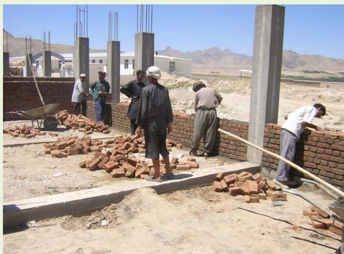
Laborers working to complete the Kohi Girls' School in August 2009. (Photo provided by SIGAR)
