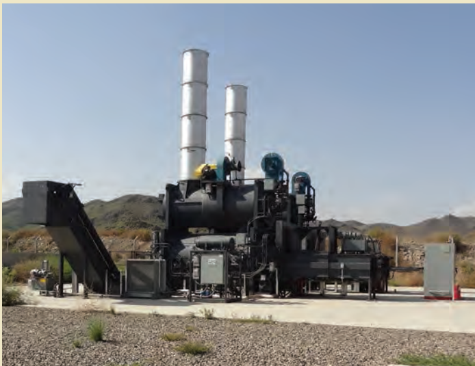
Photo 1 - Two 8-Ton Capacity Incinerators at FOB Salerno
