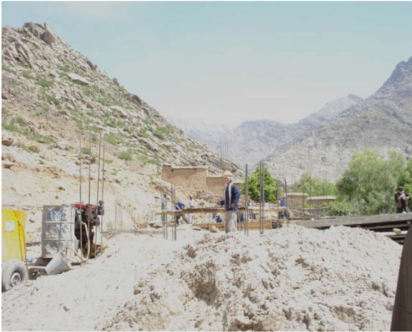
Site Photo 1: View of the challenging terrain where the Abdul Manan School is being constructed. Extensive grading work was required at this site prior to construction. (Photo provided by SIGAR)
